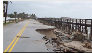
Washed out roads in Indian River County after Hurricane Frances.
